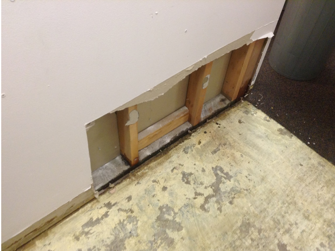
Figure 1 - "Ground Zero" for office leak (in hallway, opposite side of wall from break room)
