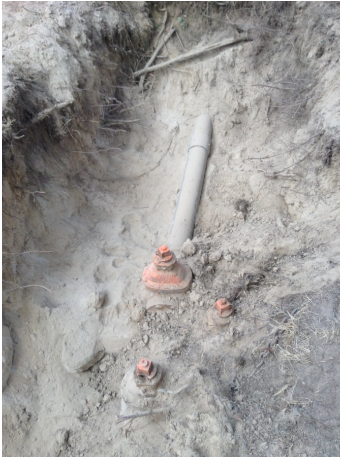
Figure 9 - Unknown Water Valves
