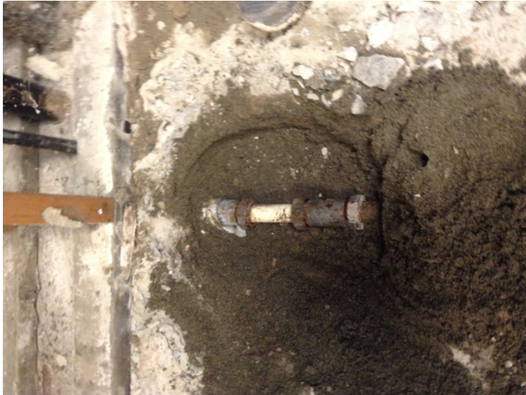
Figure 3 – Service line from main trunk to leak location (in Kitchen Area)
