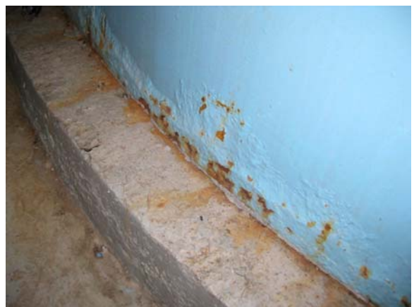
Rotoflow – Corrosion at Base
