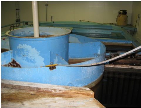
Rotoflow Package Equipment
