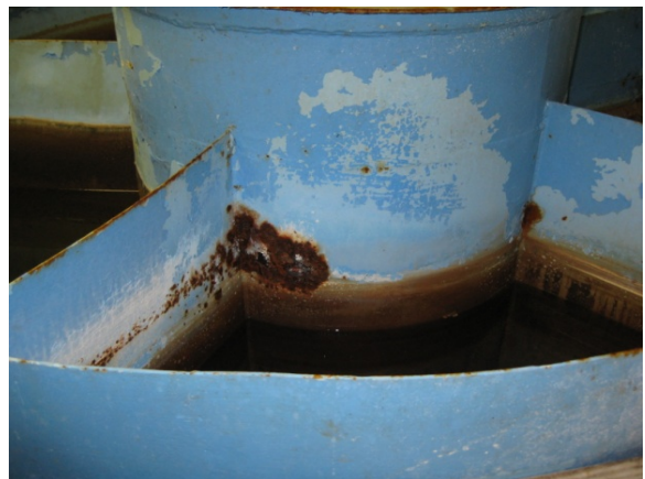
Rotoflow – Corrosion at Flocculator
