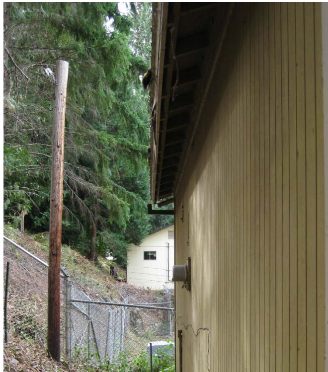
Missing Gutter at East Side of Building
