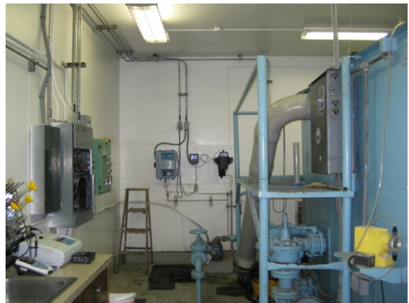
Water Treatment Plant Interior
