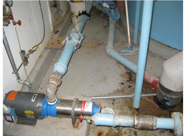
Finish Water Pump
