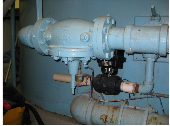
Non-Functioning and Improper Filter-To-Waste Components (white PVC, black valve)
