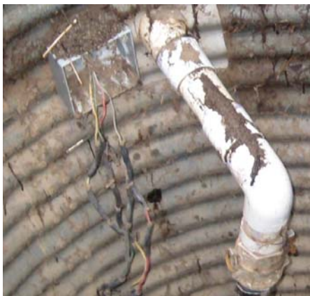
Deficient Wiring to Intake Raw Water Pump
