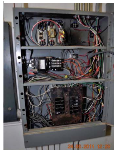
Existing Pump Control Panel
